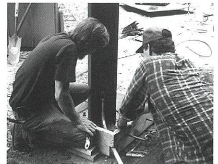
Luther Campbell and Malcolm George installed the grounding grid at the new addition of Plant No. 6. This important process will keep lightning strikes in a controlled path and minimize lightning damage.
